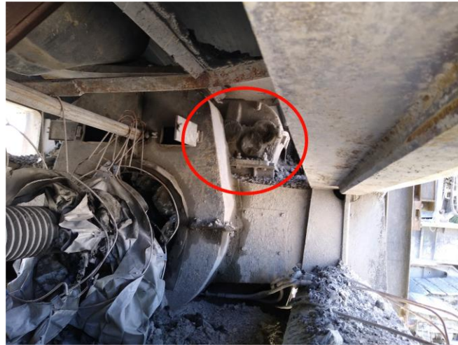
Figure 4. Interior of the chamber and position of the machine reducer.
