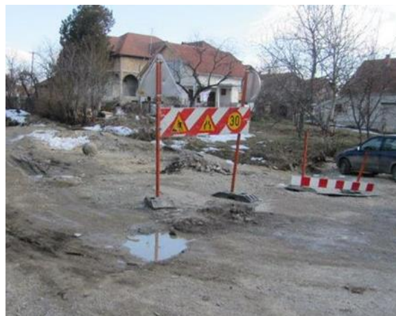
Figure 1. An example of poor regulation and direction of traffic in the roadwork zone.
